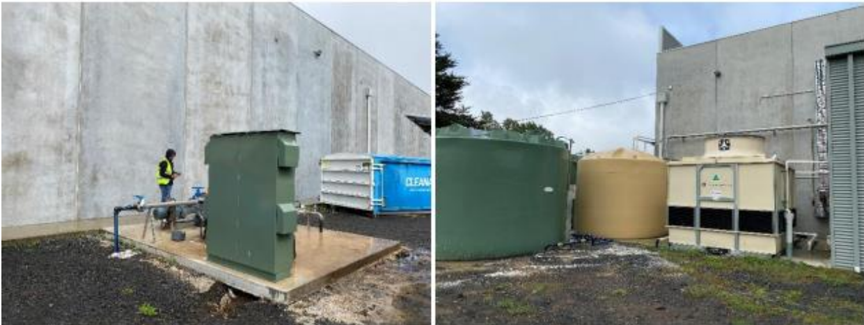
Rising Sewer Main Pump Station (left) Cooling Tower, Cooling Tower Water Tank and Effluent Waste Water Tank (right)
