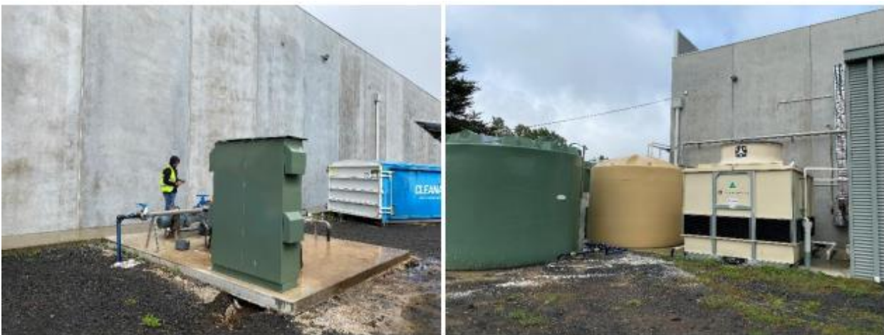
Rising Sewer Main Pump Station (left) Cooling Tower, Cooling Tower Water Tank and Effluent Wastewater Tank (right)
