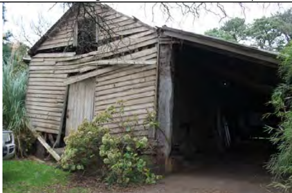
Photo 6: Outbuilding at 'Mayfield' possibly the remnants of a meeting room attached to the former Bungaree Mechanics' Institute, 2014. Source: Dennis Spielvogel.
