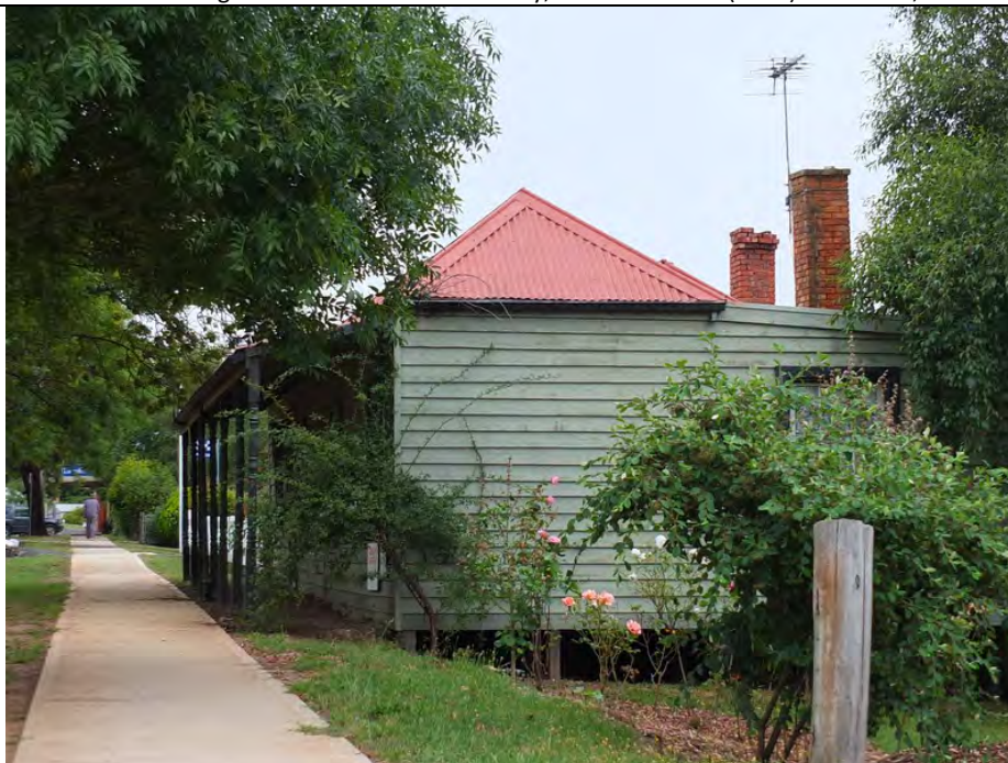
Photo 3: Dwelling and former bakery and store, east elevation showing replacement floor stumps and weatherboard wall cladding, as well as rear skillion addition, 2015.
