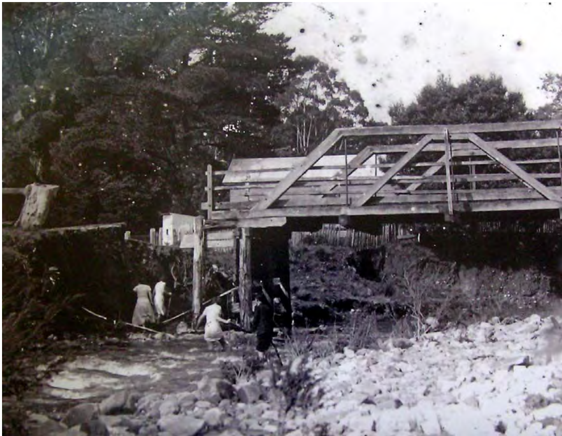
Figure 8: Damaged bridge over the Lerderberg River at the Blackwood Cricket and Recreation Ground after the flood c.1945. Source: Blackwood and District Historical Society collection.
