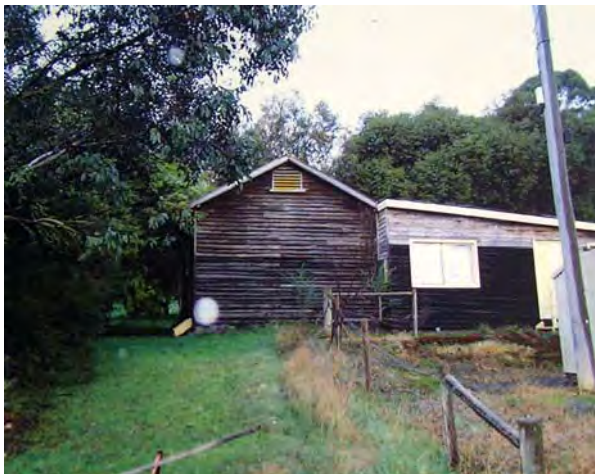
Figure 5: Former Police Stables with skillion addition, n.d. [c.1978]. Source: Crown Land file, Rs 9548 DEPI.
