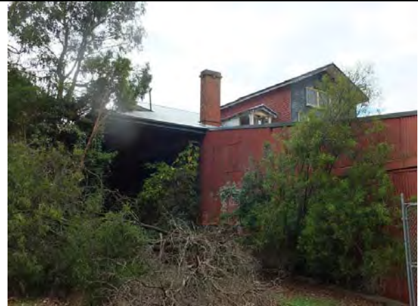
Photo 5: Former Butter Factory, south elevation, 2014. The left portion is the porte-cochere of 1908, with original chimney and small lantern light. The elevated gabled wing is the addition of the 1930s.
