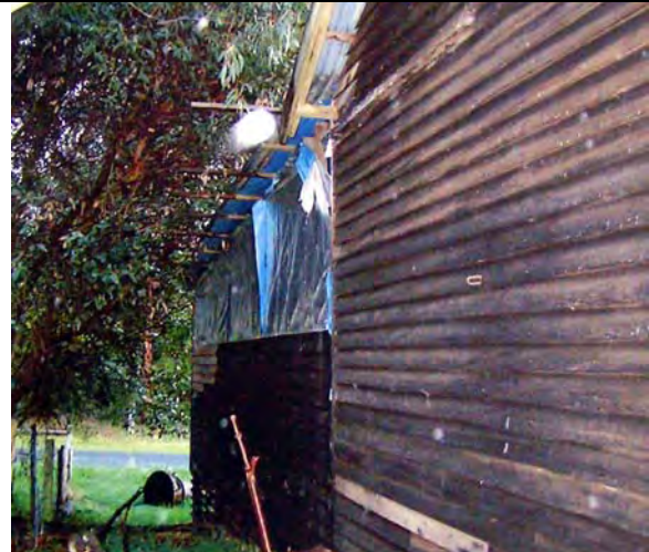
Figure 6: Former Police Stables showing skillion addition under construction, n.d. [c.1978]. Source: Crown Land file, Rs 9548 DEPI.
