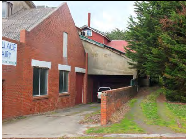
Photo 2: Former Butter Factory (Building 1), north elevation, west end, 2014. The front wing (left) is the addition of the 1940-50s, the gable end behind (with concrete infill) is the addition of 1922 and the attic gable is the addition of 1928.
