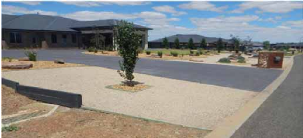
Figure 5: filled swale drain, construction of brick letterbox over nature strip and landscaping in front of a property in Mia Bella Drive, Hopetoun Park.
