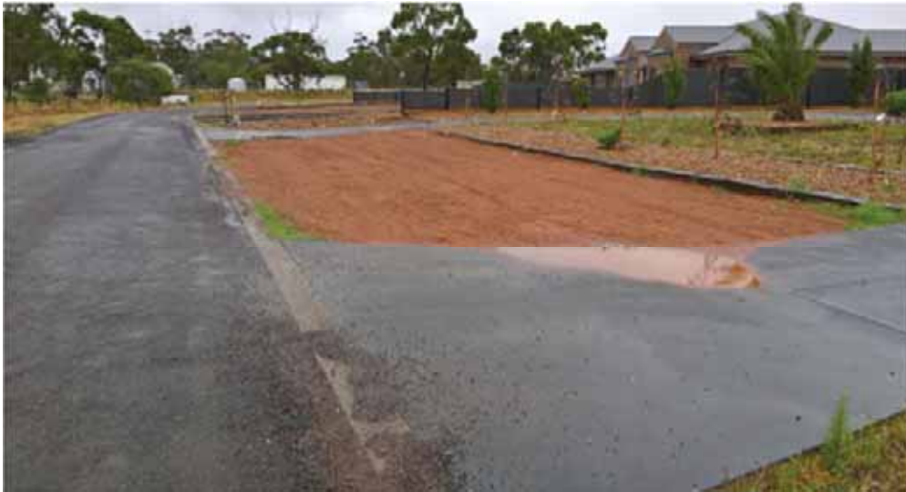
Figure 2: filled swale drain in front of a property in Carberry Drive, Hopetoun Park.
