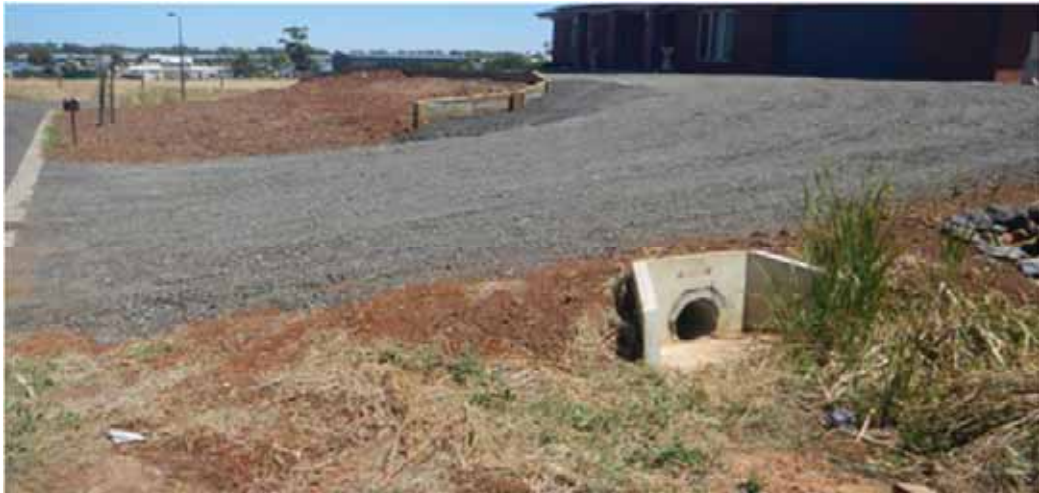
Figure 8: filled swale drain in front of a property at Eden Crescent, Hopetoun Park.
