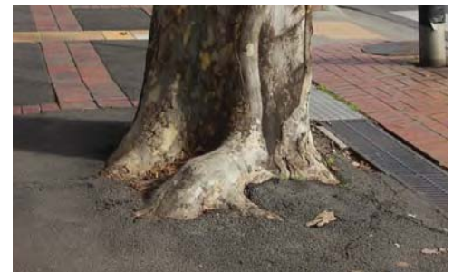
Figure 24 Root and pavement conflict
