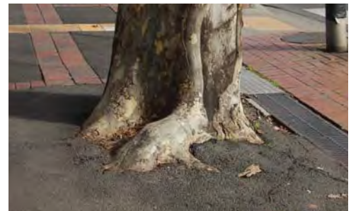
Figure 24 Root and pavement conflict
