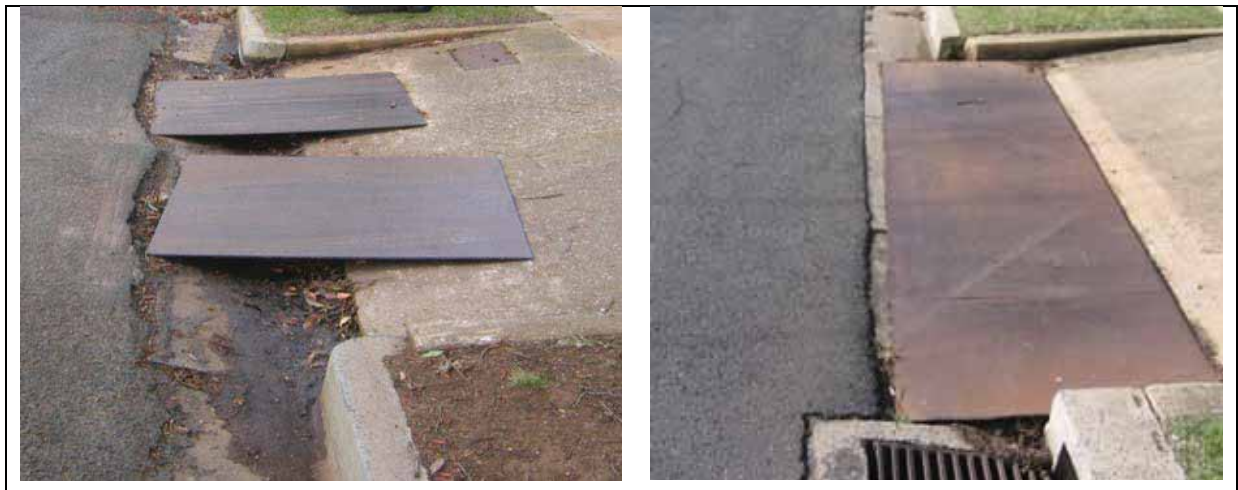
Figure 24: Problematic plated kerb ramps in Bacchus Marsh
