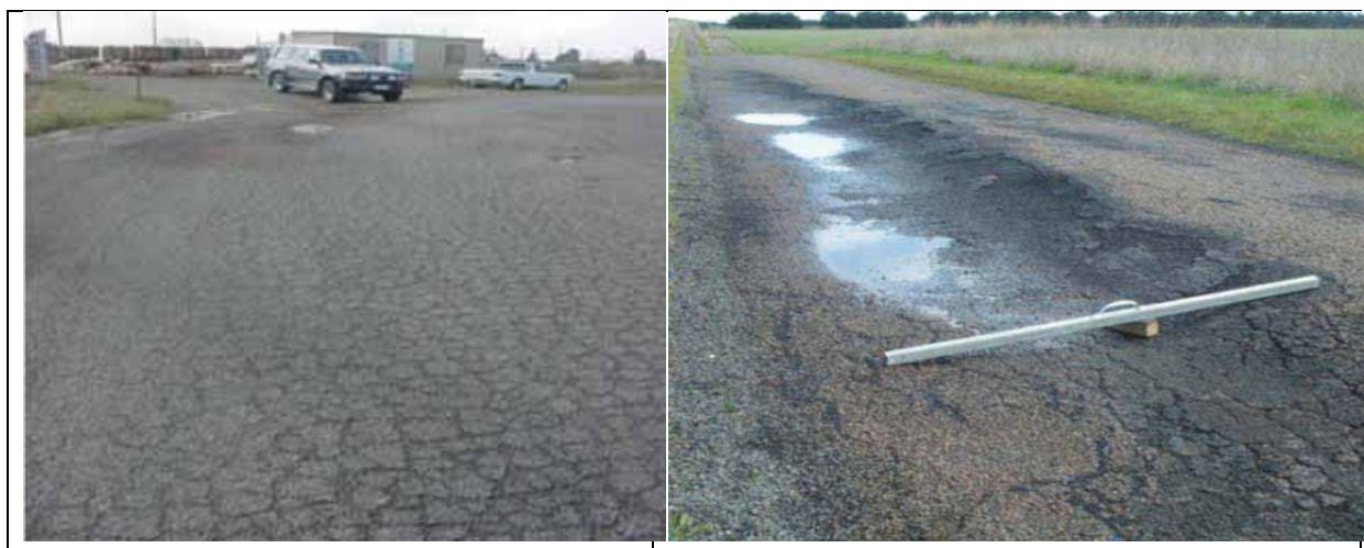
Figure 10: Examples of severe (X) & significant (#3) Cracking and Rutting
