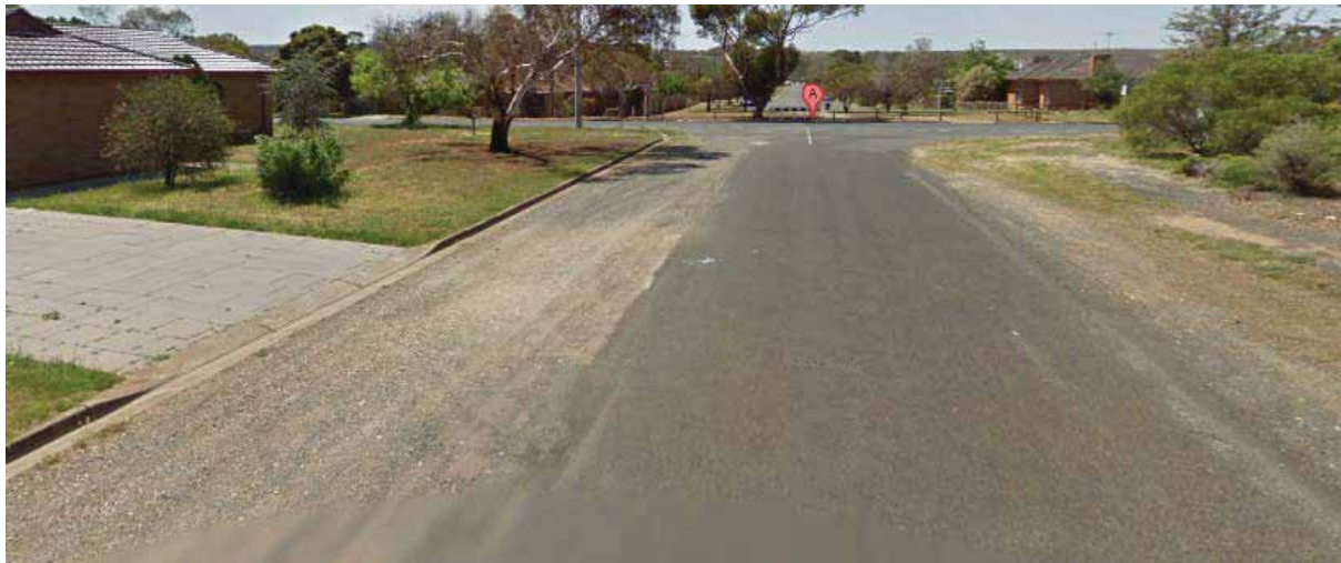
Figure 27: A bitumen strip down the centre of the road is no longer 'acceptable'
