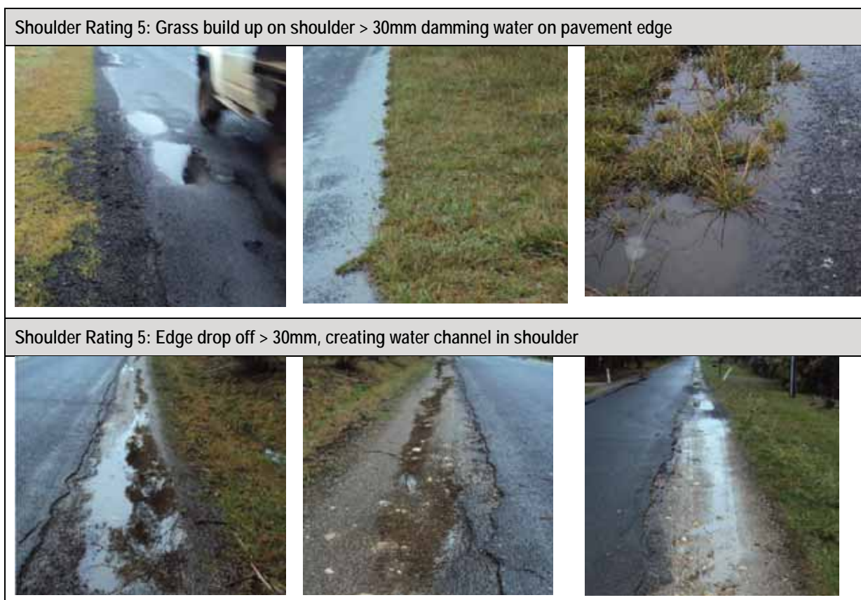
Figure 11: Examples of Shoulder Condition 'Failed'
