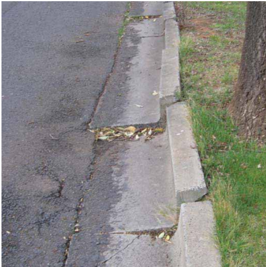
Figure 21: Legacy of past construction practices
