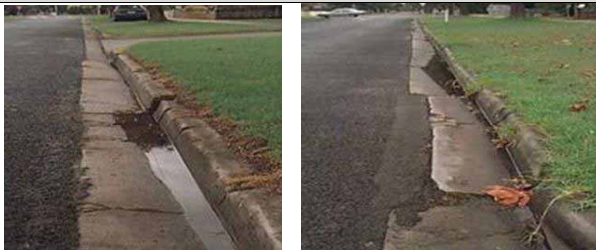
Figure 12: Examples of Kerb & Channel distress
