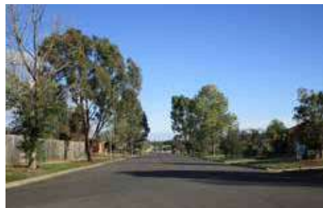
Wide road reserve, with inconsistent street tree plantings and a single sided footpath network.
